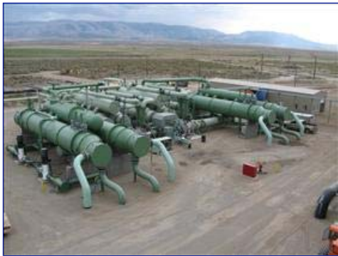
Plant and Control Room
